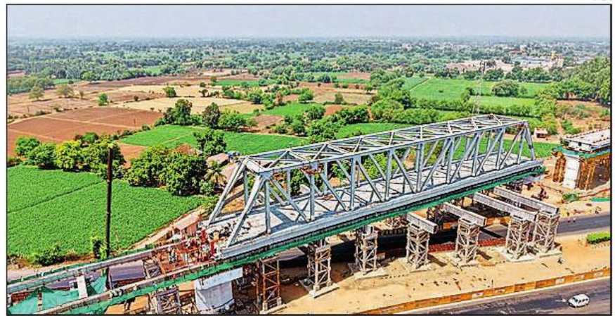
This is the first 100-metre span of a 2 X 100 metre long steel bridge
